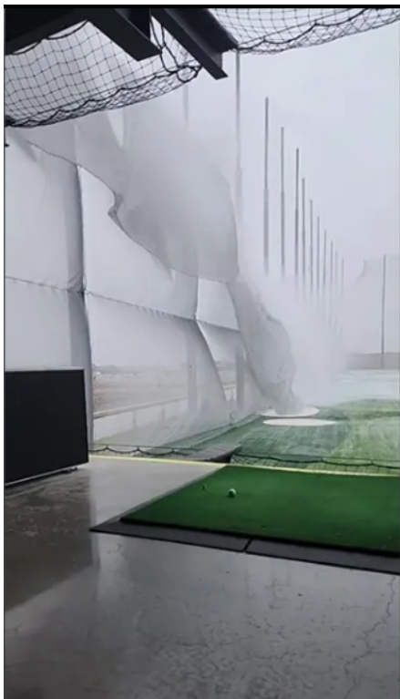
Left: Ice Accumulation causes damage to a golfing range in Fargo, ND.
